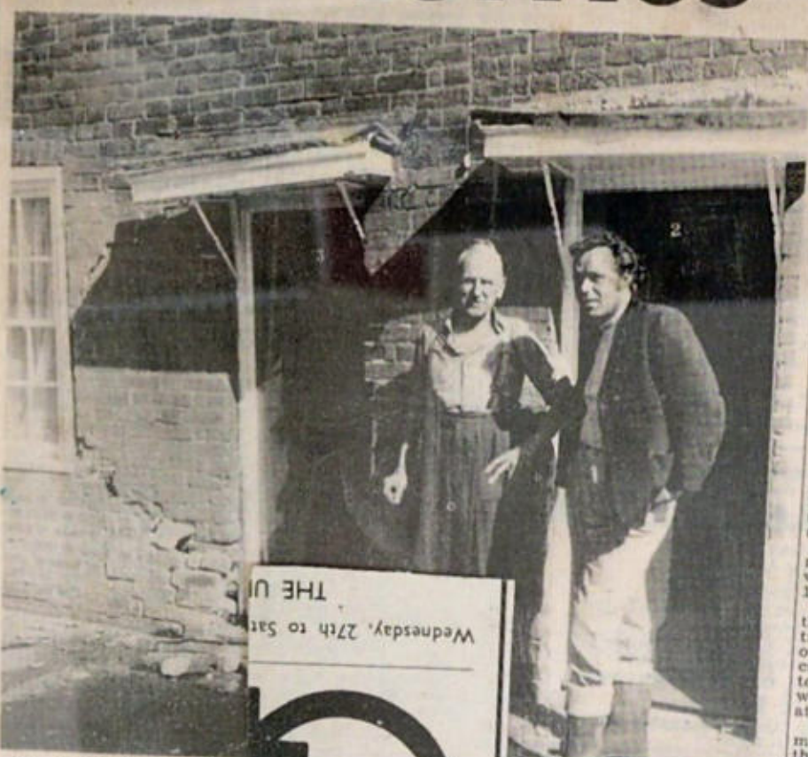
Mr. John Hatcher (right) inspects damage to 3 Hall Place Cottages, Harbledown, after a TIR lorry crashed into it on Friday. With Mr. Henry...
