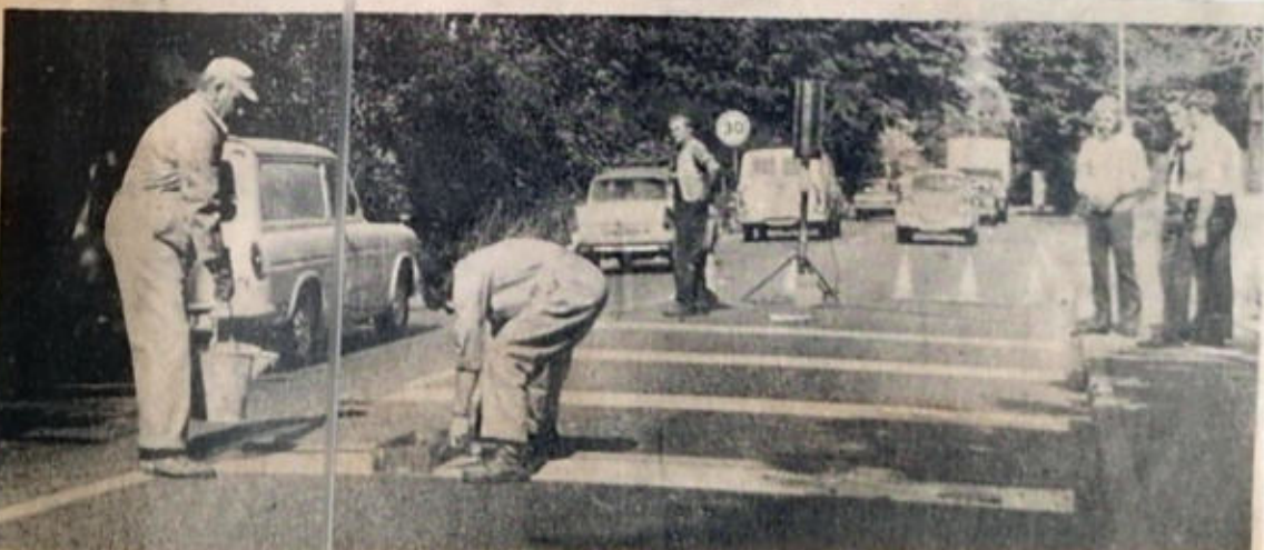
Workmen busy painting yellow lines across the A2 at Bridge on Wednesday. The lines are designed to encourage drivers to slow down.
