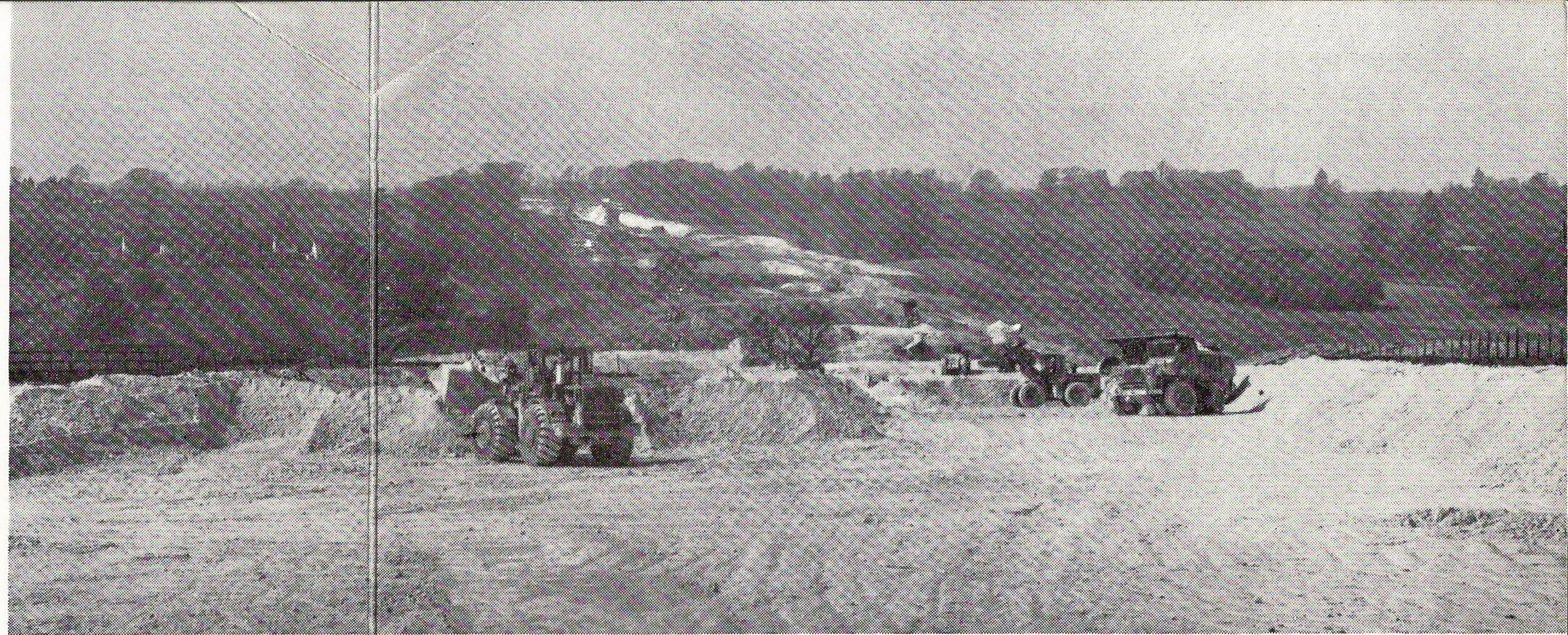
The line of the bypass is becoming apparent as teams of excavators and lorries move chalk in April 1975.
