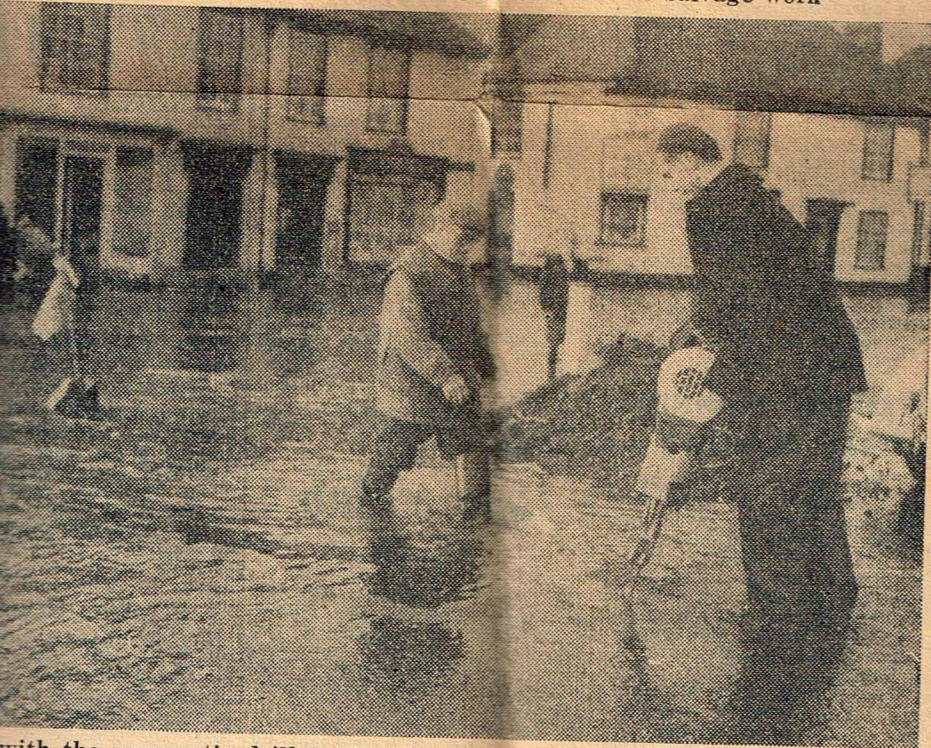
with the pneumatic drill is digging a channel at Bridge to help the water to escape . . . Background is a buoy to mark the way for motorists
