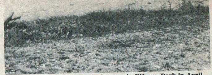
Patricxbourne bridge and the by-pass in Bifrons Park in April, 1976. Work was forging ahead by then, as the men got ahead of their time schedule.
