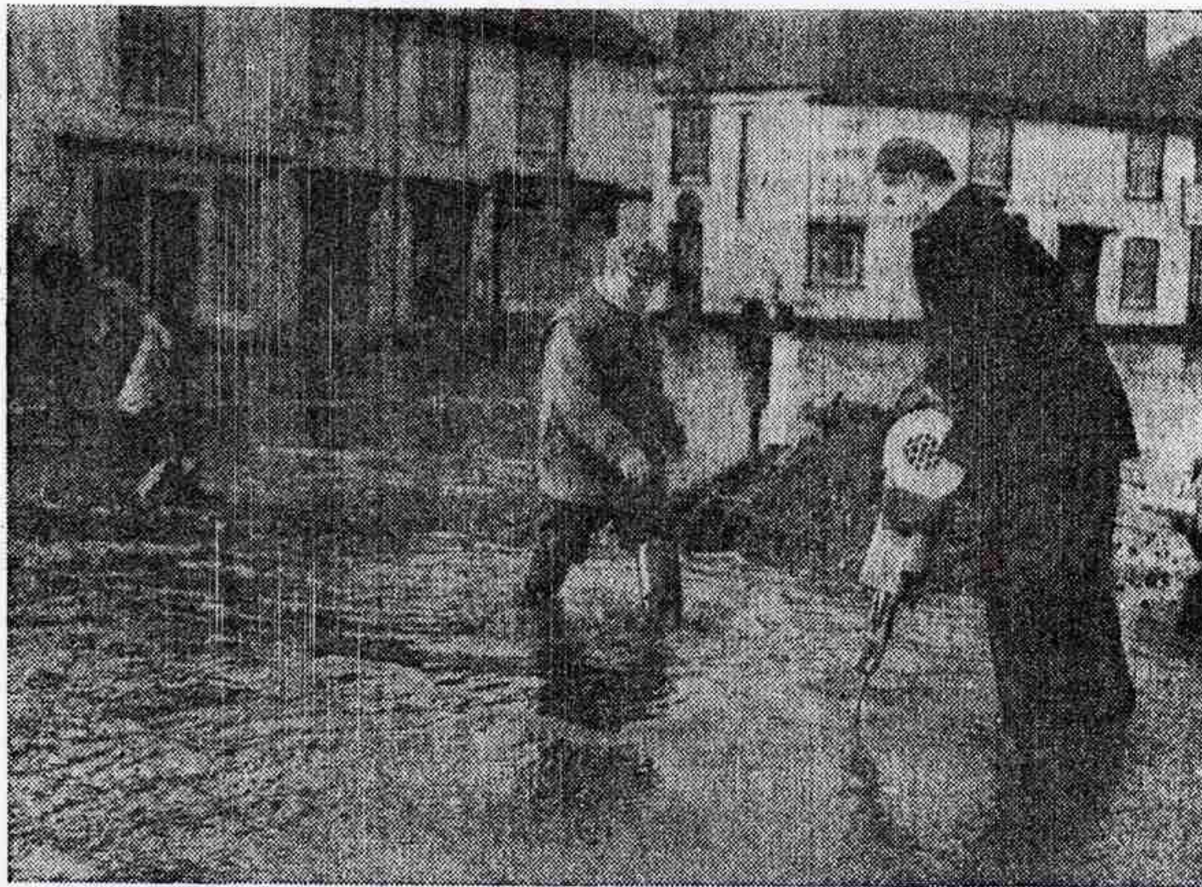
Man with the pneumatic drill is digging a channel at Bridge to help the water to escape . . . Background is a buoy to mark the way for motorists
