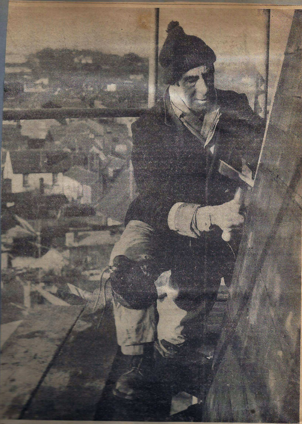
Over 120 feet above the rooftops of Bridge works Mr. L. Thorner, of Folkestone. For the last week he has been retiling and slating the village church steeple.
