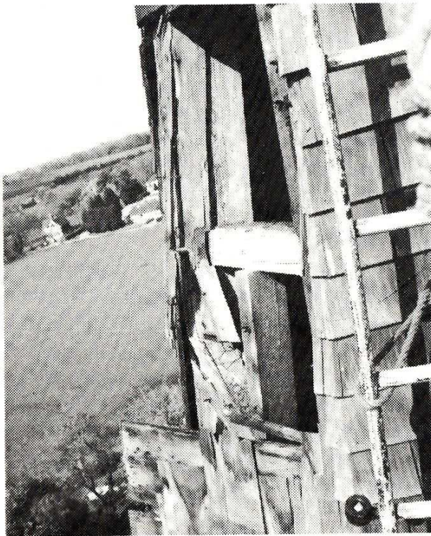
Some of the damage in close-up.
