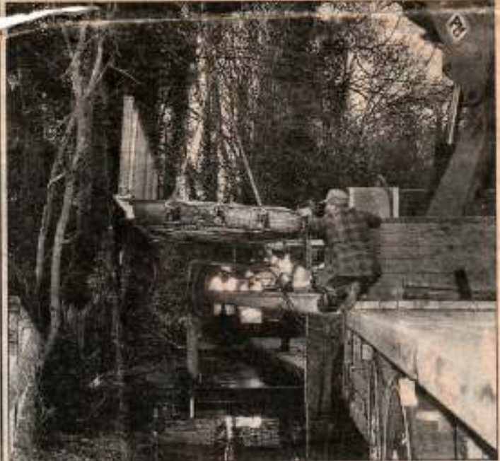
ON LOCATION: Workers place the temporary bridge over the ford in Rose Lane
