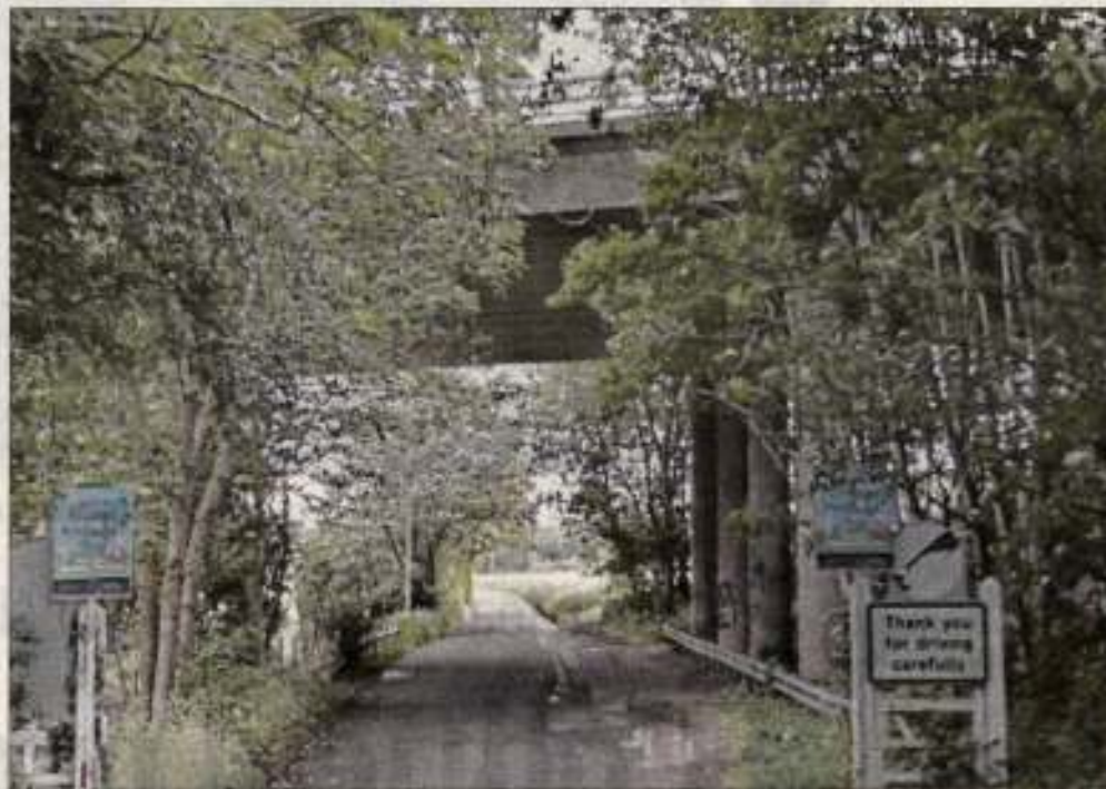
The bridge which carries the A2 over Patricxbourne Road in Bridge, Canterbury is to have 24 bearings replaced in essential maintenance work
