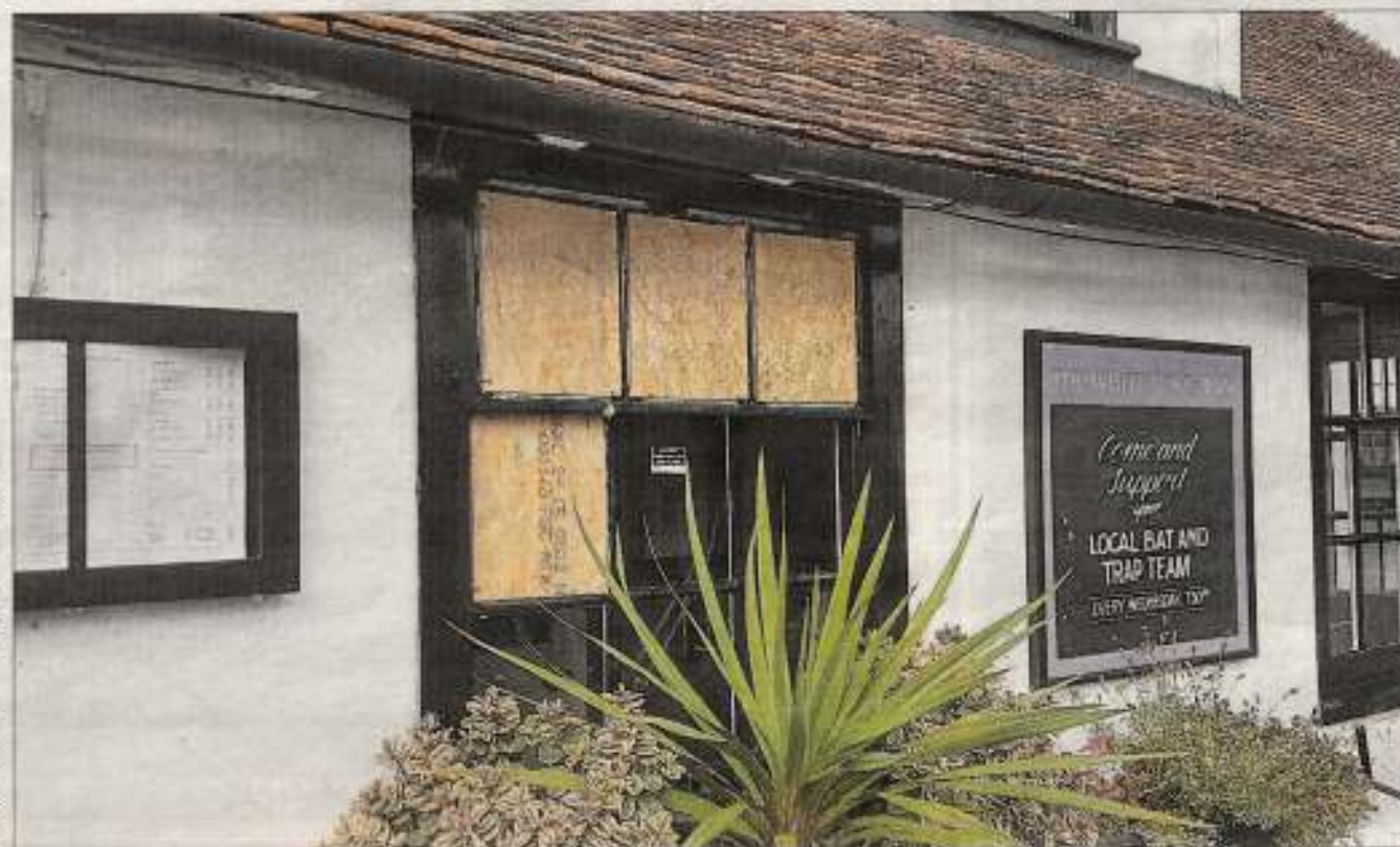
Windows have been boarded up following the vandalism at the White Horse Inn in Bridge
