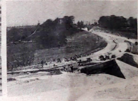
Pairixbourne bridge and the by-pass in Bifrons Park in April, 1976. Work was forging ahead by then, as the men got ahead of their time schedule.
